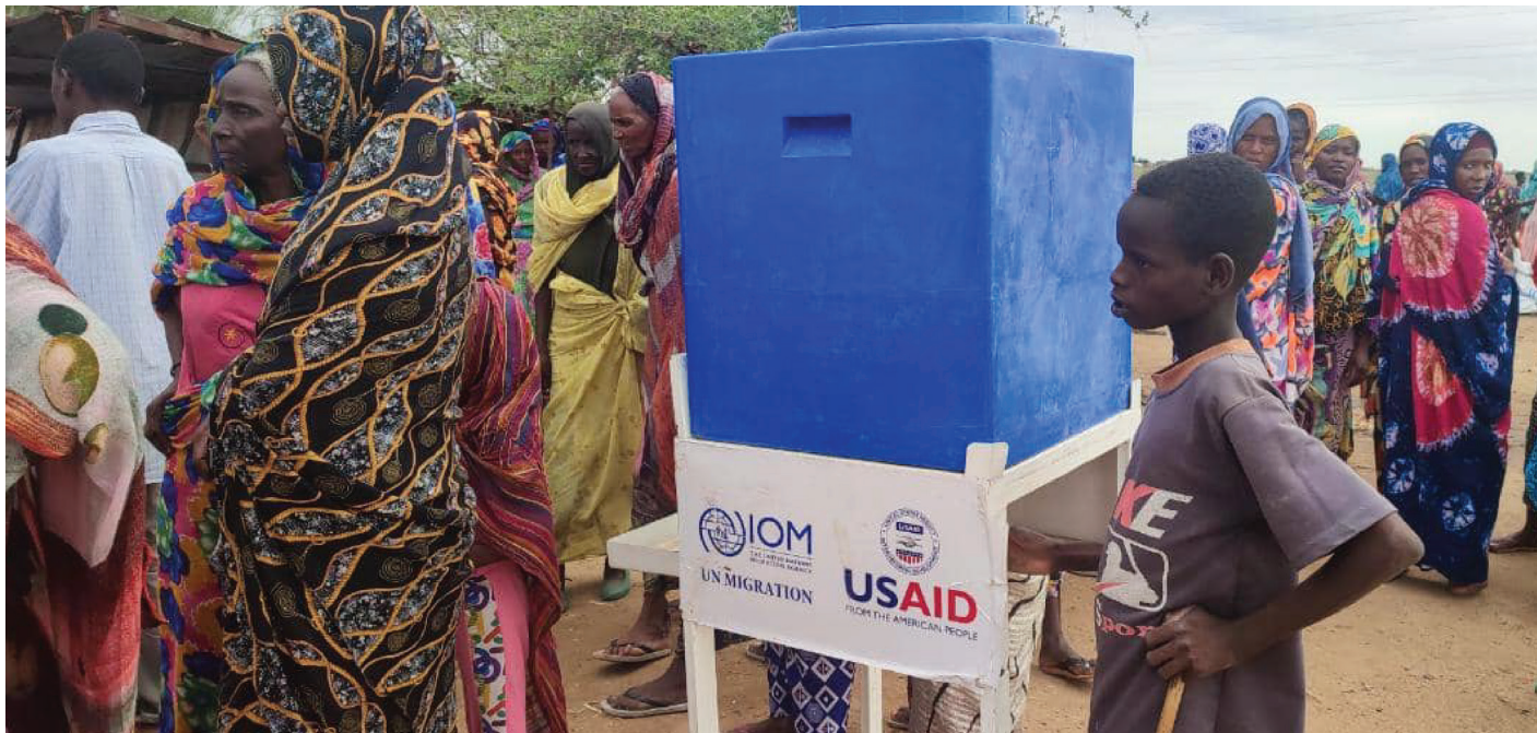
Portable handwashing facilities installed in Blue Nile Region. IOM 2023
